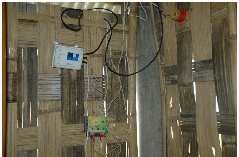
Early warning receiving unit at at Dihiri along Jadhah River (Dhemaji District). Credit: ICIMOD
