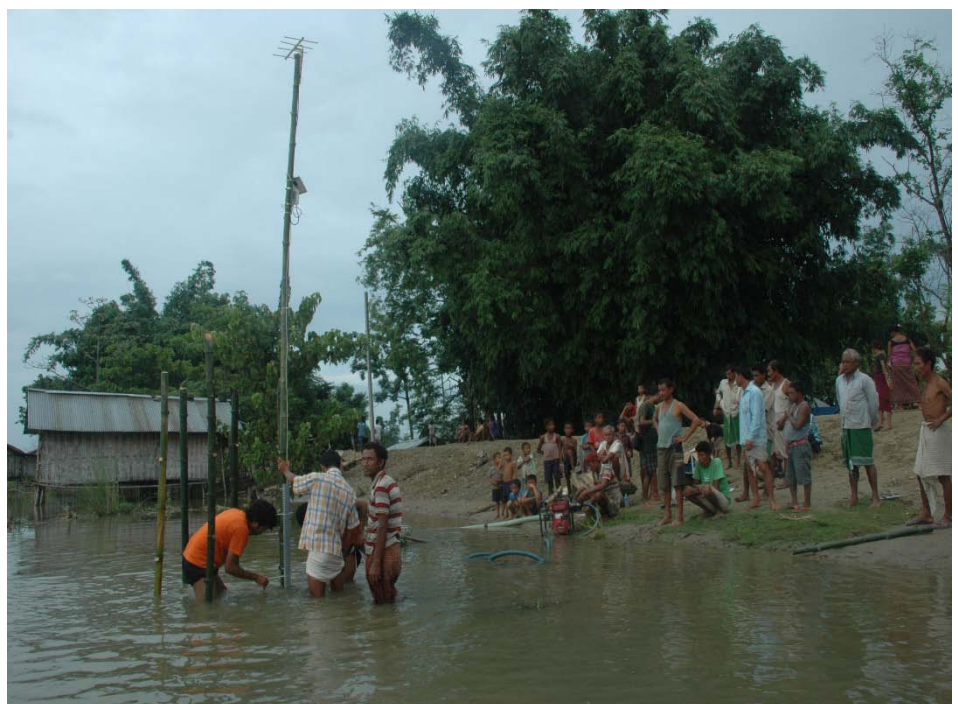
Flood early warning system installation at Dihiri along Jiadhah River (Dhemaji District). Credit: ICIMOD
